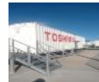
ENEL Green Power (Italy) 4MW-1MWh TERNA Virtual Storage Plant (Italy) 1MW-1MWh
